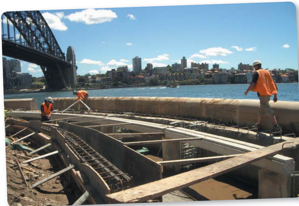
Dawes Point Seawall is being restored, preserving a precious piece of Sydney's history
